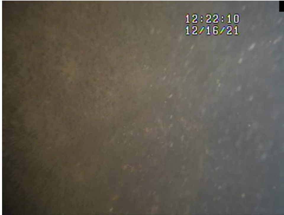
Figure 2 - Concrete Sill: Marine Growth
